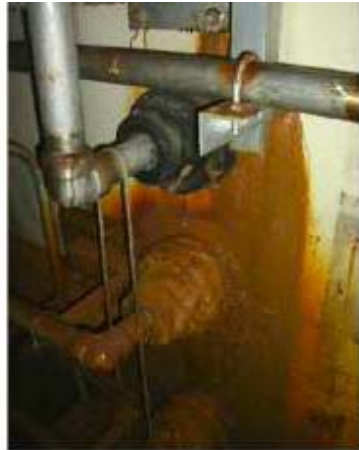
Water flowing in from where the pipe penetrates through the wall
