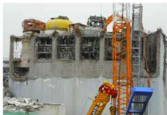
After debris removal (Upper part of the operating floor, west surface) Photo taken on July 9, 2012
