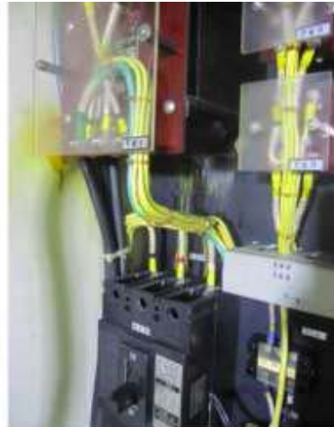
Location where smoke was coming out from (inside the control panel)
