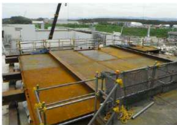
Protection platform installation on the Spent Fuel Pool Photo taken on June 15, 2012
