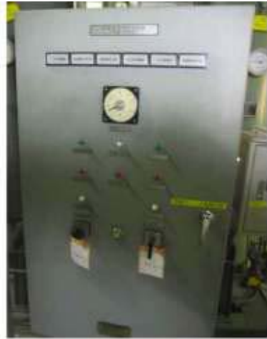
Control panel of the compressed air system (IA system)
