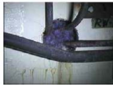
⑤ Water exuded on the location where the pipe penetrates through the south wall of the spent sludge tank A
