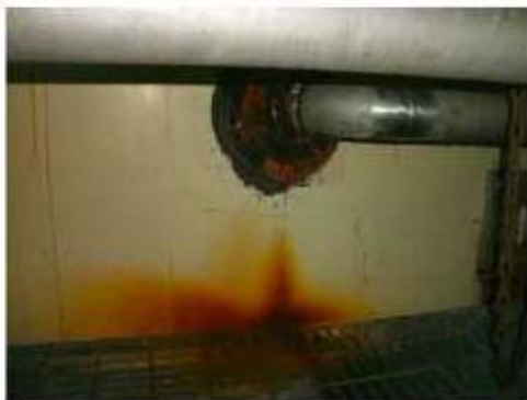
1. Location where water flow was confirmed on Unit 2 Offgas Pipe Duct
