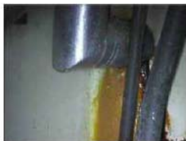
① Location where water flow was confirmed on the Centralized Environment Facility Radiation Waste Common Duct (Water amount: Width of 3 fingers, No change)
