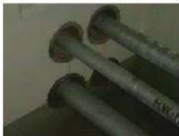
③ Location where the pipes penetrate through the wall between the reactor coolant filtering system spent resin storage tank room and the spent sludge storage tank room (under the water)
