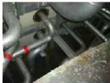
④ Location where the pipes penetrate through the wall between the radiation waste underground storage facility building and the radiation waste treatment building (under the water)
