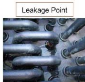
Air Fin Cooler B2: 2 points leakage Air Fin Cooler B3: 2 points leakage
