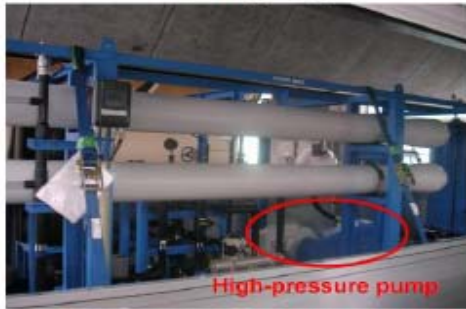
Reverse osmosis membrane in reverse osmosis membrane unit
