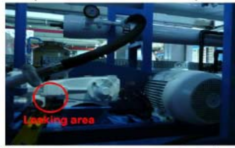
High-pressure pump in reverse osmosis membrane unit
