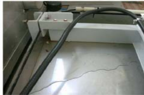
Status of leakage (before wiping off)
