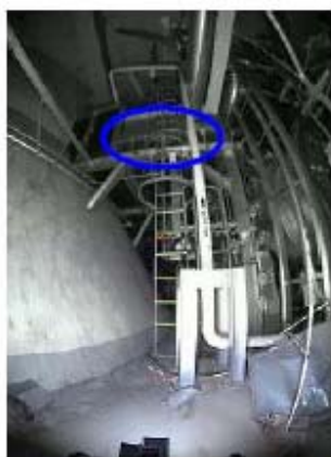
Grating at the valve of Core Spray System
