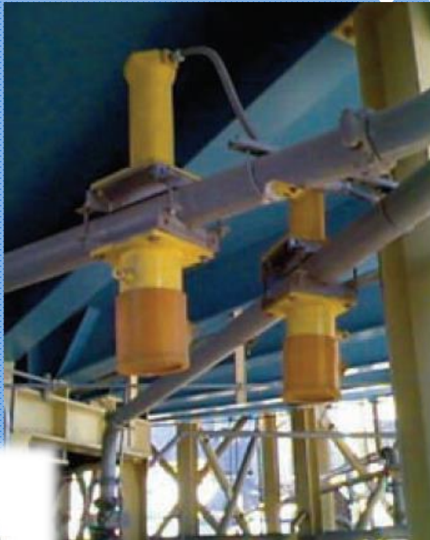
FIG. 66. Pipeline density gauges in position.
