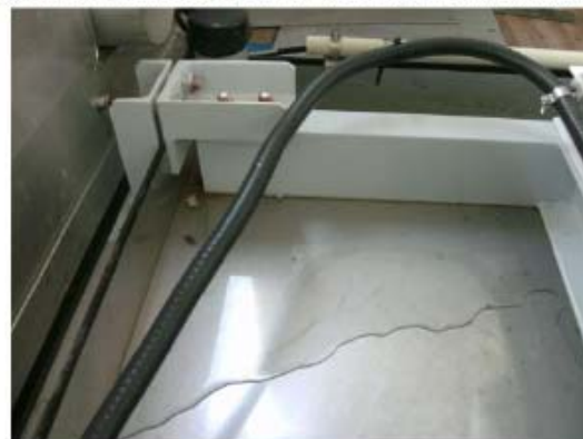
Status of leakage (before wiping off)
