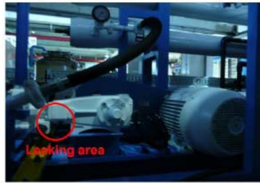
High-pressure pump in reverse osmosis membrane unit
